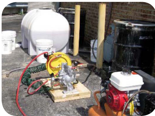
ISCO system installed behind a small drycleaning facility.
